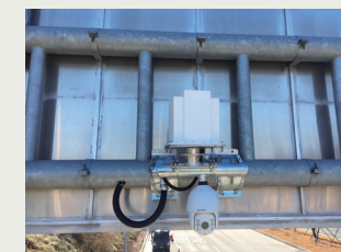
돌발상황검지시스템(AIDS) Automatic Incident Detection Systems
